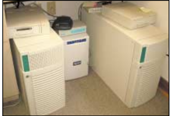
Fig. 7 Two computer servers, battery backup, KVM switch, tape backup drives, modem for Kodak OrthoTrac Classic access, and Internet modem.
